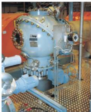
Filter type PR-BW 100 in a power plant
